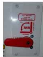
Water Heater Bypass
