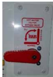
Water Heater Bypass
