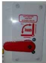
Water Heater Bypass
