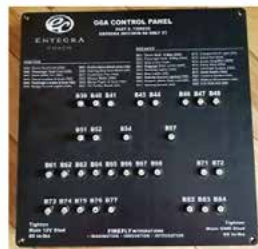
GFCI Breaker Panel
