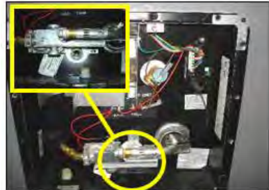
Fig 1: Water Heater Drain Plug
