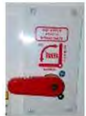
Water Heater Bypass Valve
