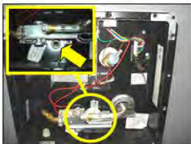
Water Heater Drain Plug
