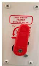
Water Heater Bypass
