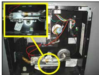
Water heater drain plug
