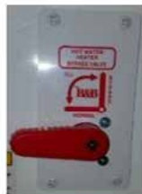
Water Heater Bypass
