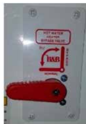
Water Heater Bypass
