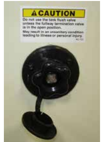
Tank Flush Inlet
