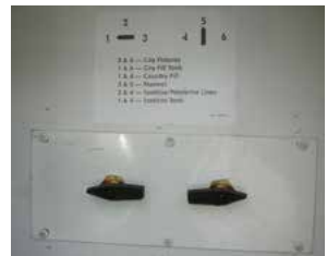
Fig. A -Water Valve Controls
