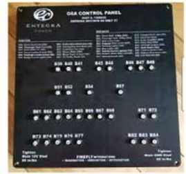
GFCI Breaker Panel
