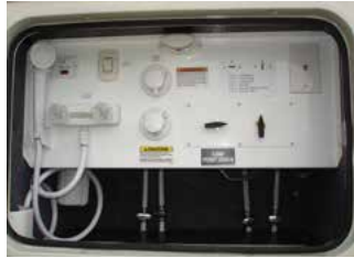
Fig. B - Utility Center
