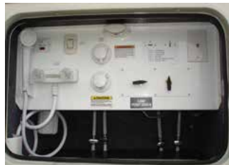
Fig. B - Utility Center
