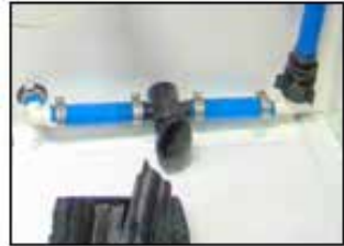
Water supply shutoff to the cartridge water filter (shown OFF)
