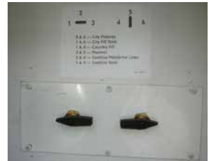
Fig. A -Water Valve Controls
