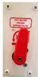
Water Heater Bypass
