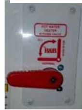
Water Heater Bypass
