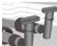
Low Point Drains
