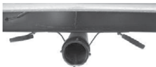
Black/Grey Tank Drain and Valves
