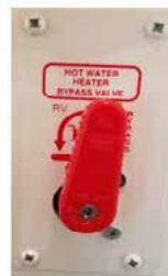
Water Heater Bypass
