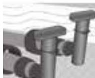
Low Point Drains
