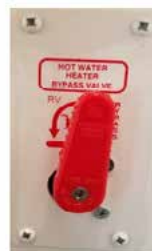
Water Heater Bypass
