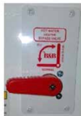
Water Heater Bypass
