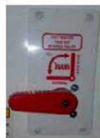
Water Heater Bypass
