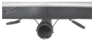
Black/Grey Tank Drain and Valves
