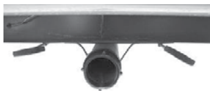
Black/Grey Tank Drain and Valves
