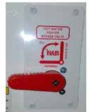
Water Heater Bypass
