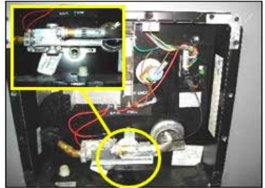
Water Heater Drain Plug
