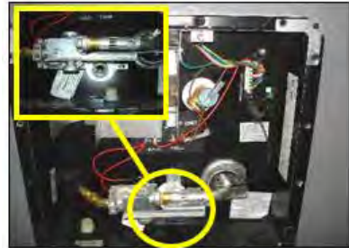
Fig 1: Water Heater Drain Plug
