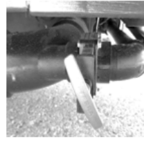
Grey Tank Drain
