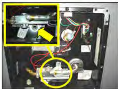
Water Heater Drain Plug
