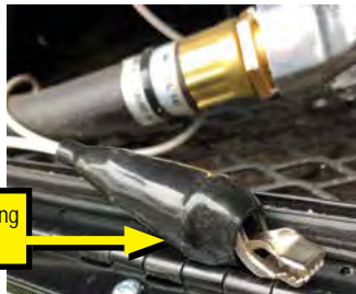
Grounding Clip Inside Fuel Station
