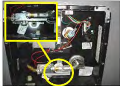
Fig 1: Water Heater Drain Plug
