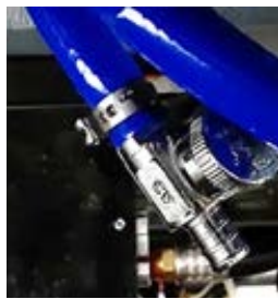
Fresh Water Drain Valve
