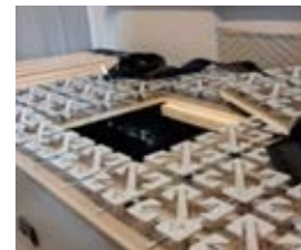
Water Heater Bypass Access
