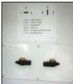
Fig.A - Water Valve Controls
