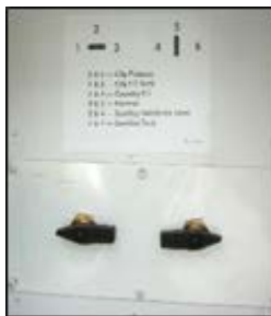
Fig.A - Water Valve Controls
